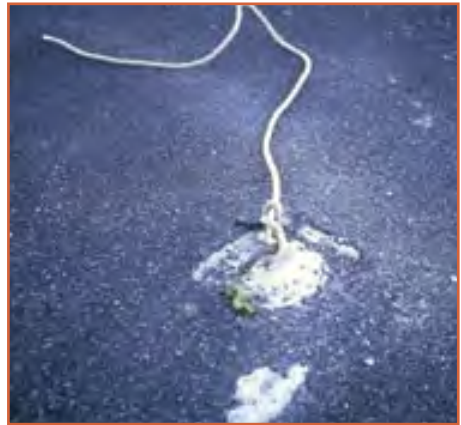
Fixed tiedown anchor point.
